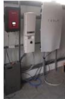
Microgrid and storage
